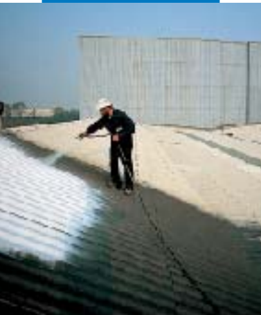
Spraying Aquaflex onto corrugated asbestos cement after treating with Primer for Aquaflex
