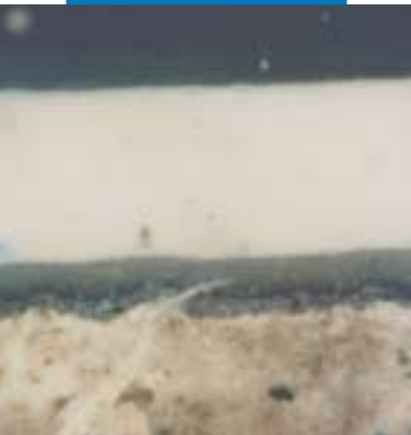
This picture highlights both the penetration of the primer into the asbestos cement as well as the efficiency of the encapsulation of the asbestos fibres which is already guaranteed by the primer
